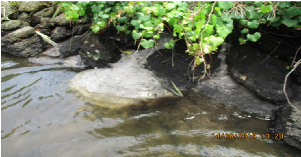
Photo 2 - Sand at toe of rip rap.
